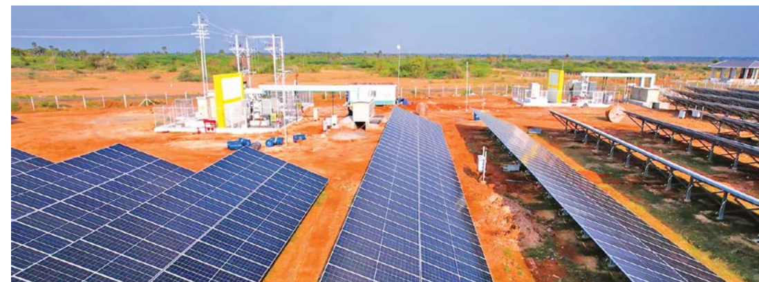
16 MWp solar PV project site in Sivagangai, Tamil Nadu, India set up by our subsidiary First Energy
