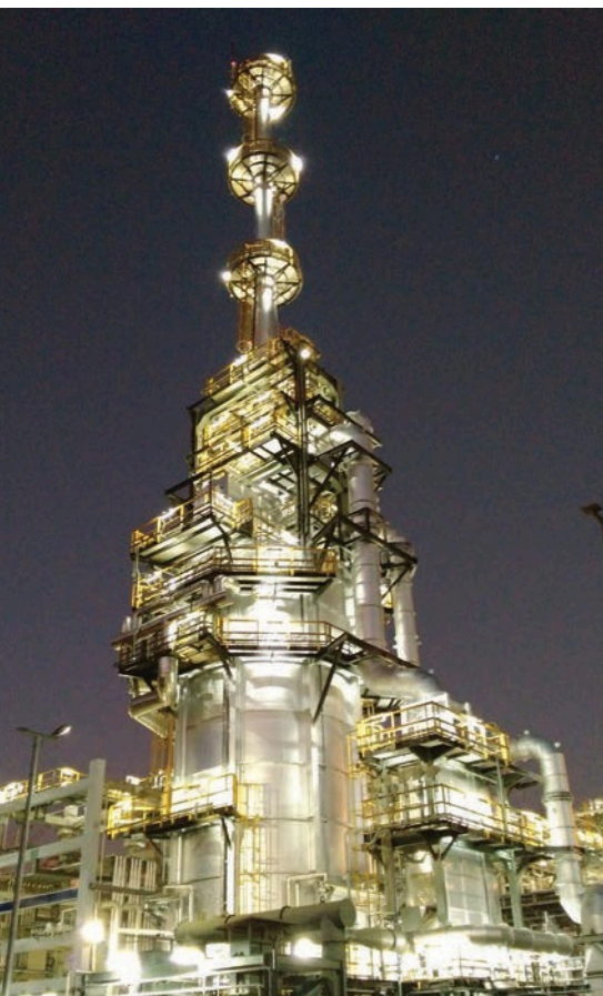
2 units of 6.34 MMKcal/hr hot oil heaters
