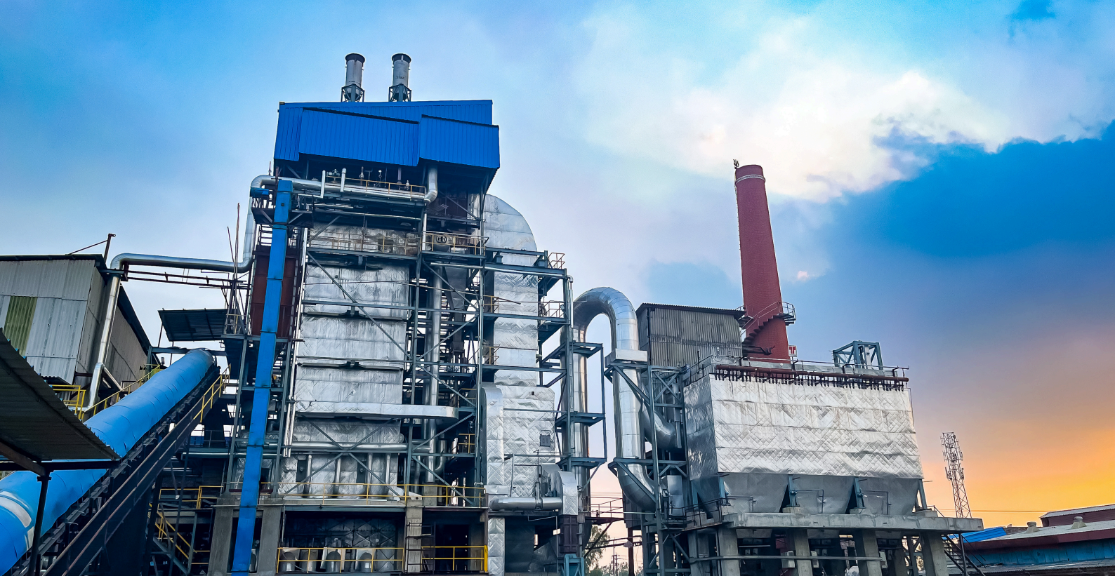
1 unit of WTE FlexiSource™ boiler in India
