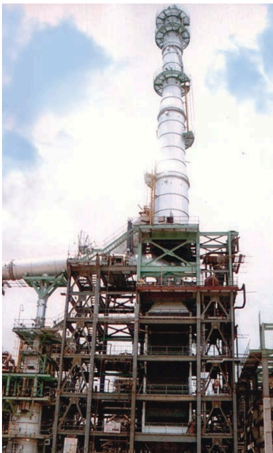
1 unit of 13.5 TPH, 30.5 kg/cm 2 g, 280°C, out board steam generator on cracking furnace
