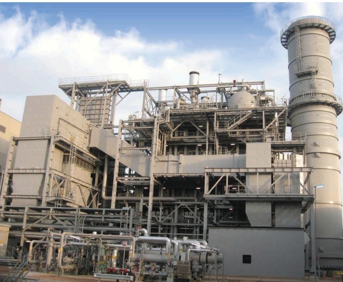
1 unit of 405 TPH, 83 kg/cm 2 (g), 310°C, natural gas, associated gas + Fresh Air Fired (FAF) boiler
