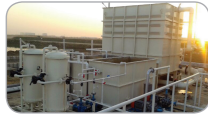
Biofilter | Low sludge sewage treatment plant
