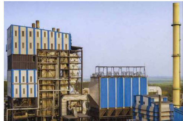
The 220 TPH CFBC boiler installed for a paper manufacturer in South India
