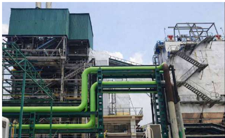
The 40 TPH AFBC bi-drum boiler installed in South India
