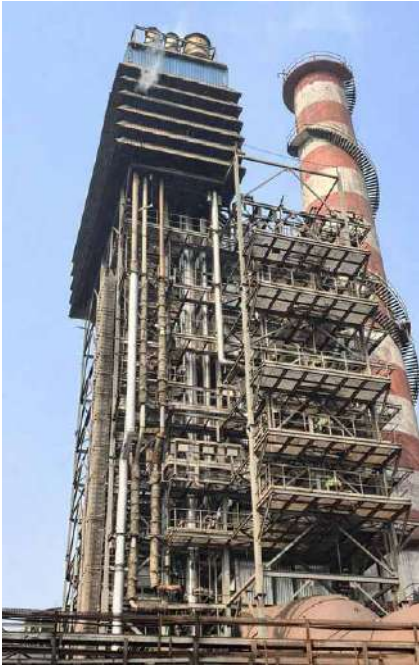
The WHRBs installed for the steel industry in Eastern India
