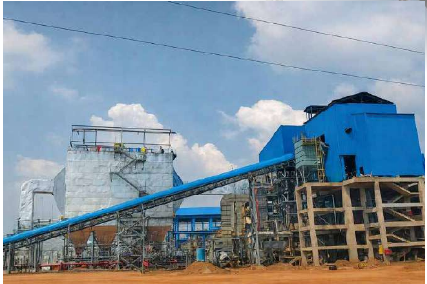
The 6.05 MW cogeneration power plant installed at Nellore, Andhra Pradesh
