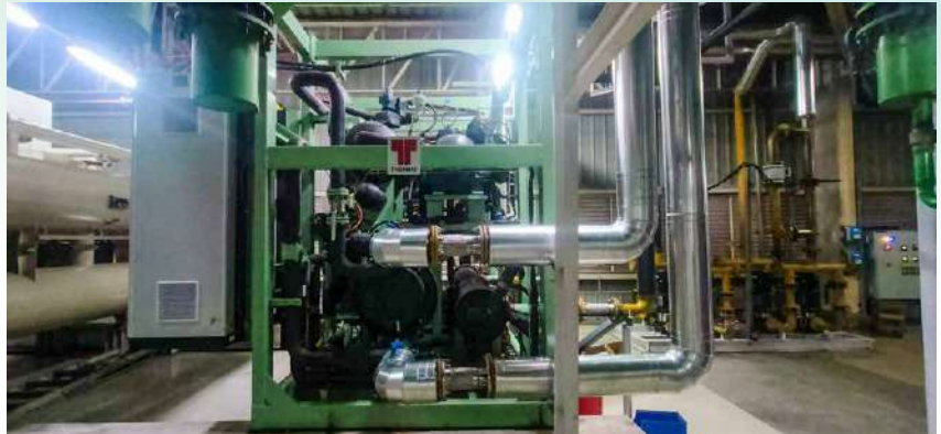
The high-temperature electrical heat pump installed at the Chakan industrial area
