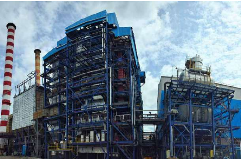
The 90 TPH reciprocating grate boiler in South India
